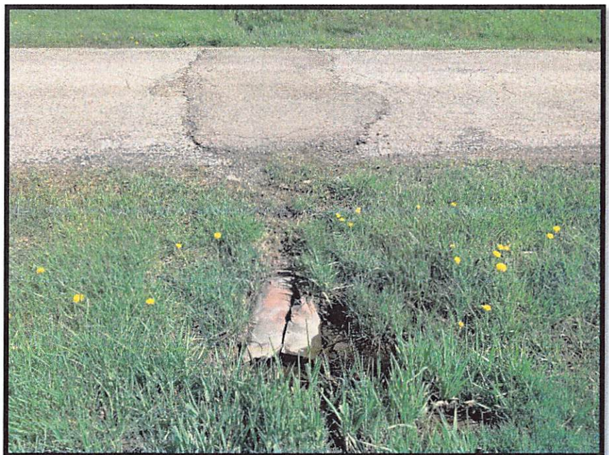
Damaged culvert under access drive – facing N
